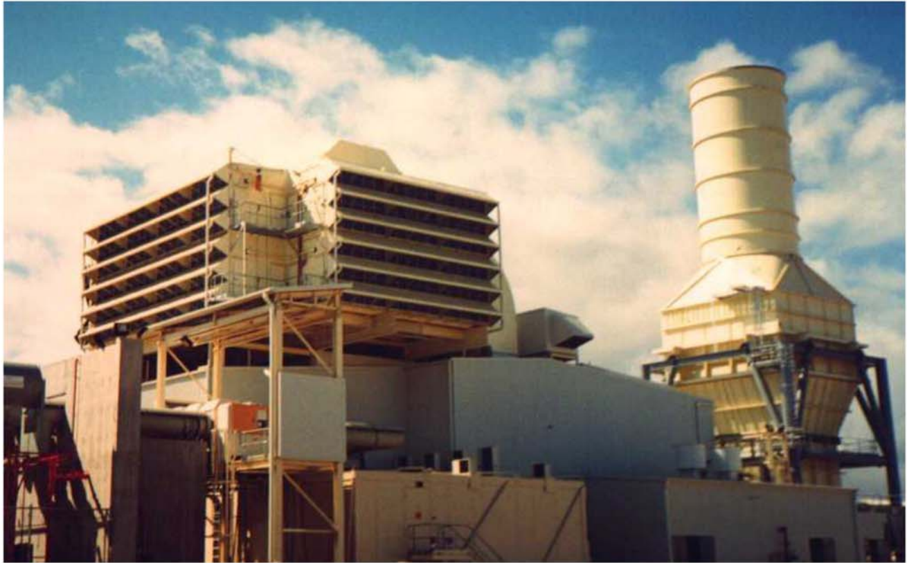
Gas Turbine Enclosure
