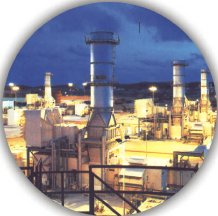
Gas Turbine Exhaust By-pass systems at Salalah, Oman
