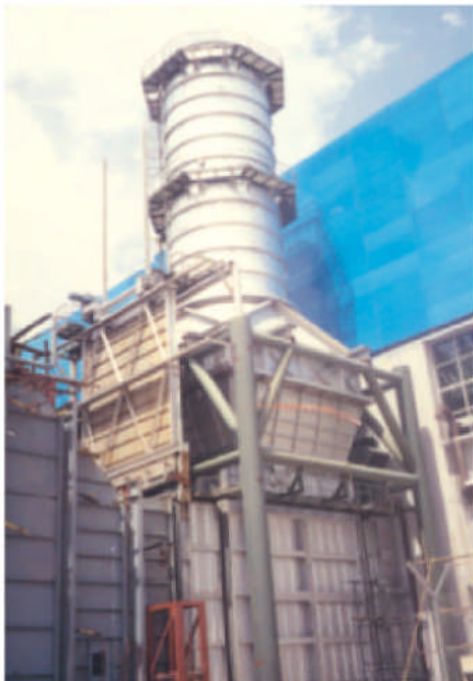
Exhaust By-pass system at Konadapalli for GE Frame-9E GT
