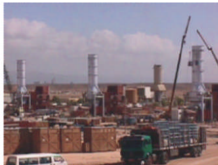
Frame-6 GT Exhaust By-pass systems at Salalah Power Station, Oman
